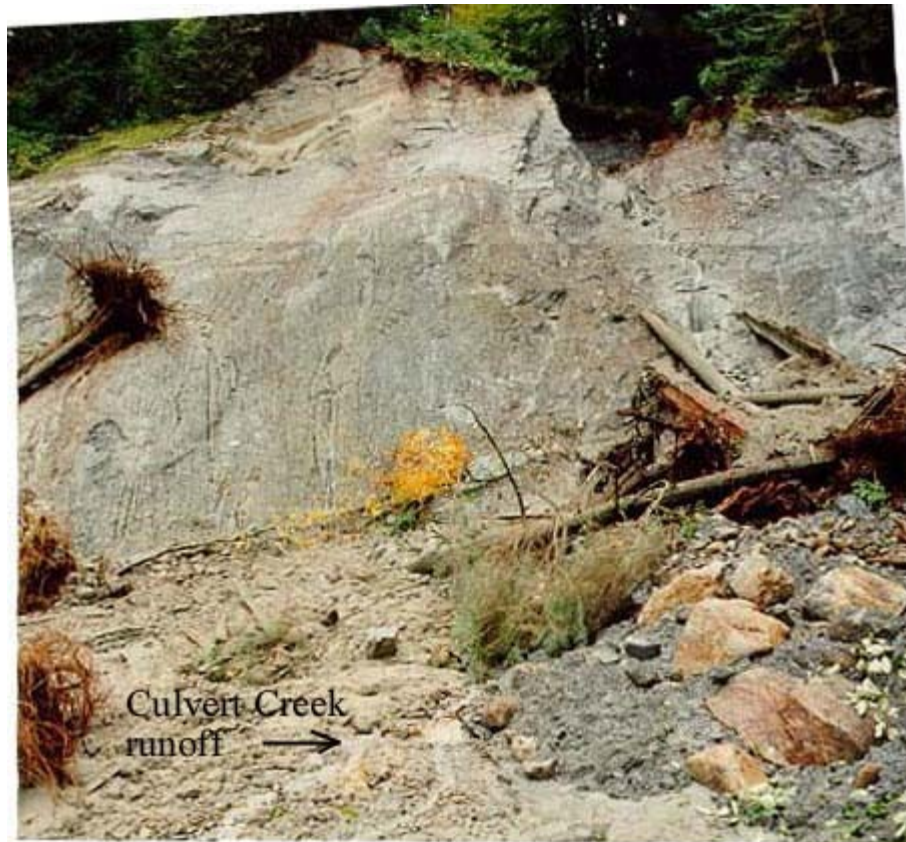
Looking up at the landslide site from Switchback Creek. Top right area shows pocket erosion created by the branch of Culvert Creek.
